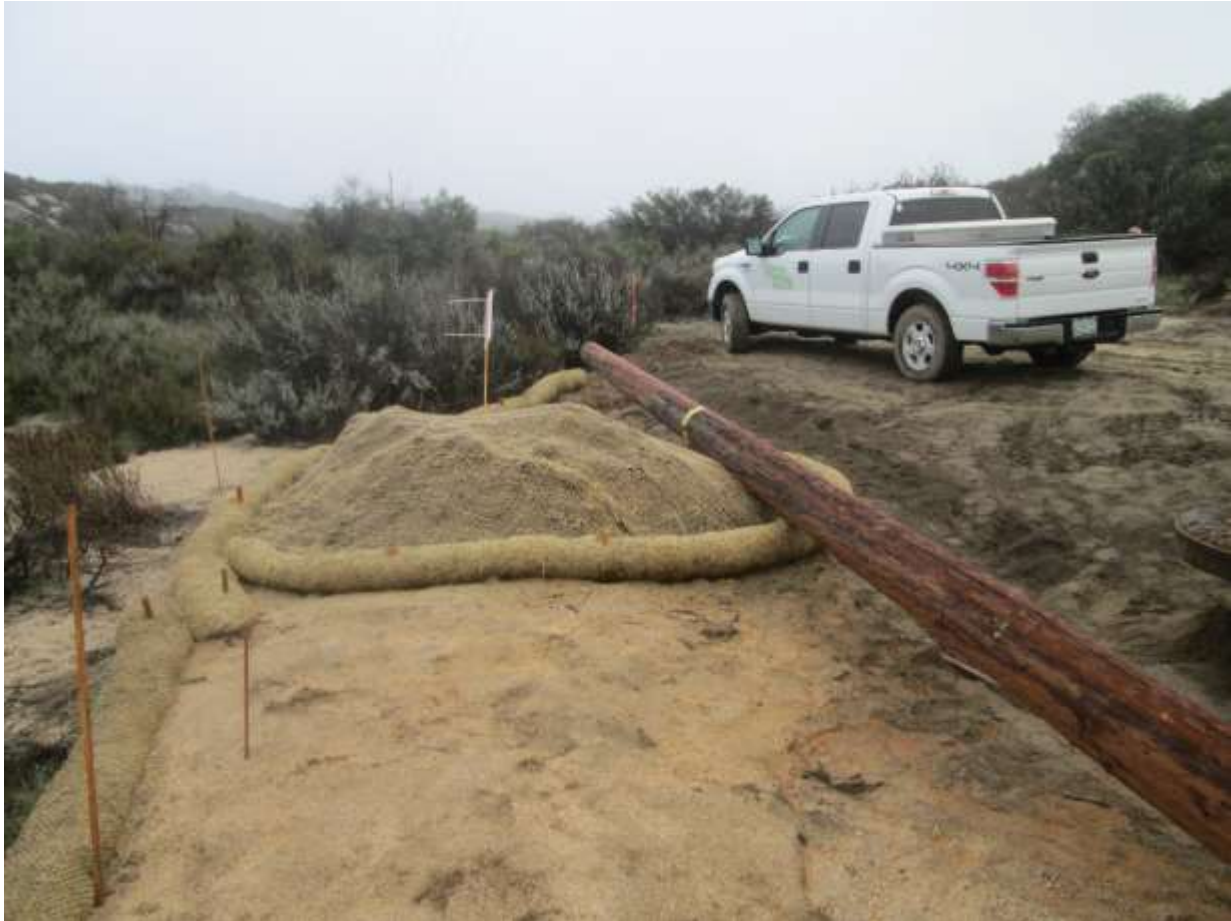
Photo 3: Topsoil was salvaged and secured within pole work area Z44184 (TL 629E), utilizing jute netting and straw wattles in accordance with the Erosion Control Plan and SWPPP as specified in the Habitat Restoration Plan (MM BIO-4).
