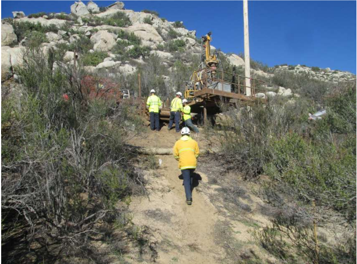
Photo 6: During equipment delivery to a helicopter micropile site along TL 629E (Pole Z44166, above), fire patrols were present in accordance with the CFPPP (MM FF-1).
